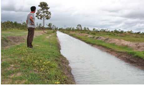
10 Km of canal digging by land recipients in Kampong Thom for sustainable agriculture production using food for work supported by GIZ-WFP cooperation
